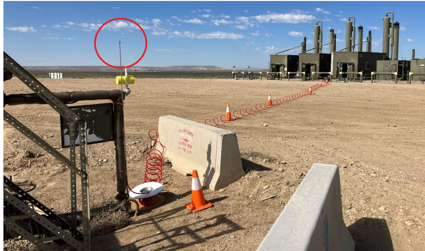
Figure A.5: A challenge release emission point during the campaign located adjacent to a wellhead and supplied gas from the challenge release rig located across the production pad near dehydration and separation equipment.
