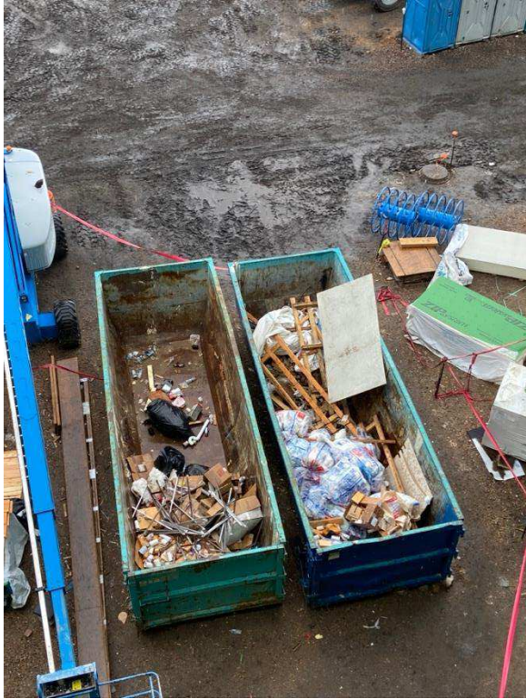
Figure 13 Wood waste in landfill dumpster (July 2023).
