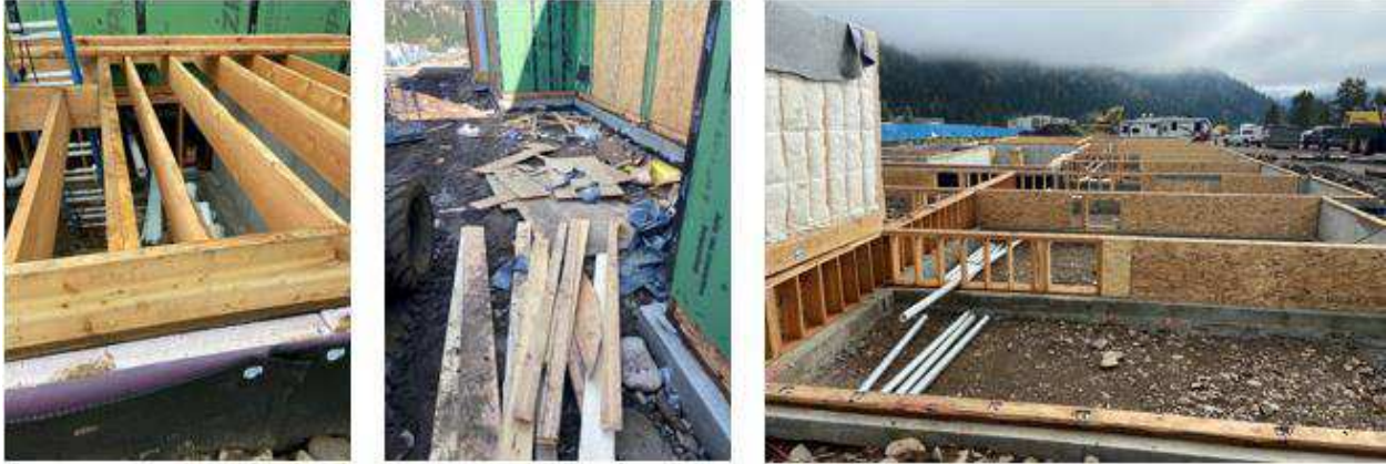
Figure 24 Observed onsite wood construction and waste
