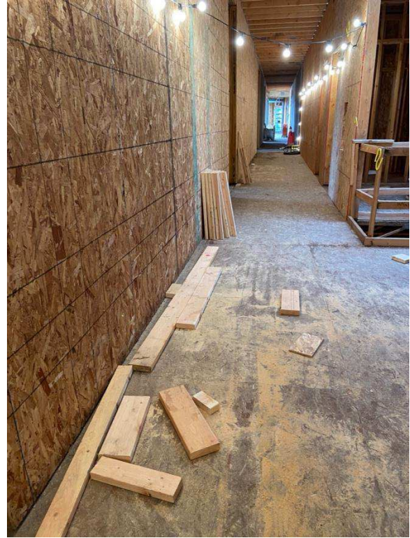
Figure 14 Wood waste on 4th floor (July 2023).
