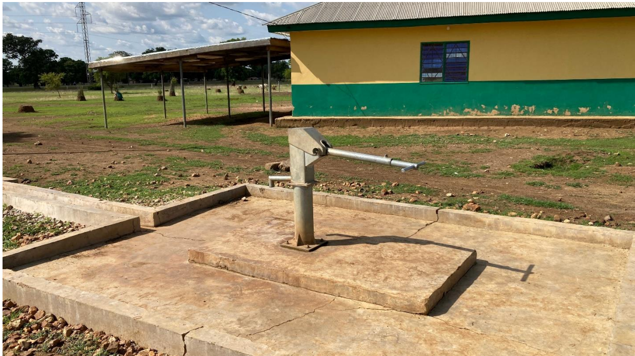
Figure 4. One of Savannah's manual pump boreholes with trough for livestock drinking.
