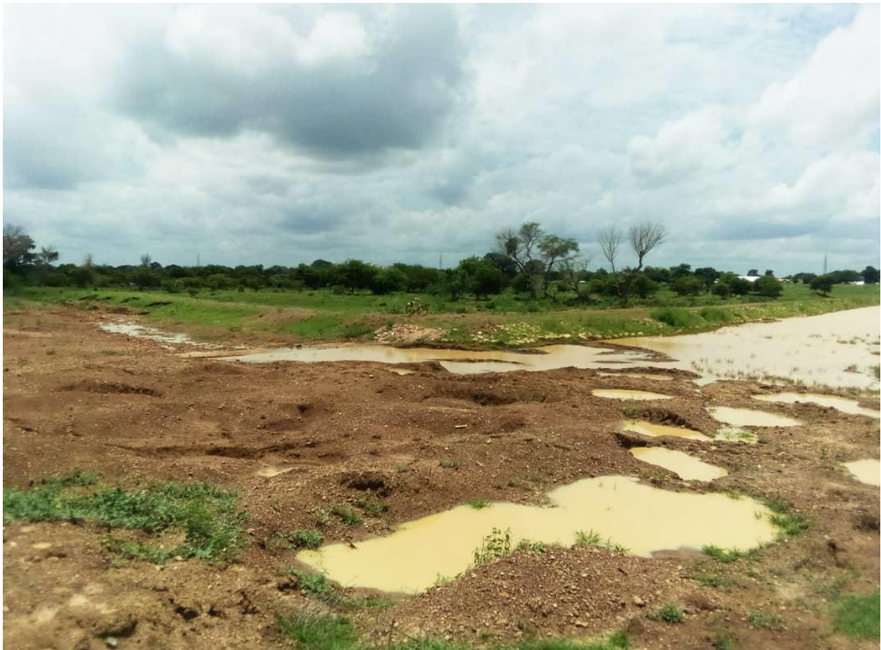
Figure 10. Galamsey pits adjacent to dam and spillway in mid-August 2022.
