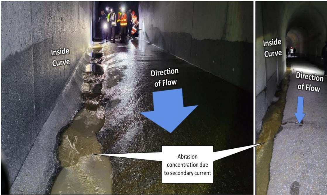
Figure 7. 2024 views of abrasion observed along the inside of a bend in the SBT at Solis, Switzerland.
