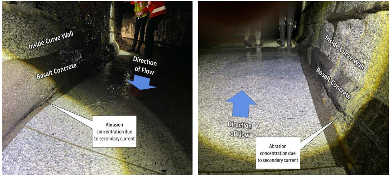
Figure 6. 2024 views of abrasion observed along the inside of a bend in the SBT at Pfaffensprung, Switzerland.
