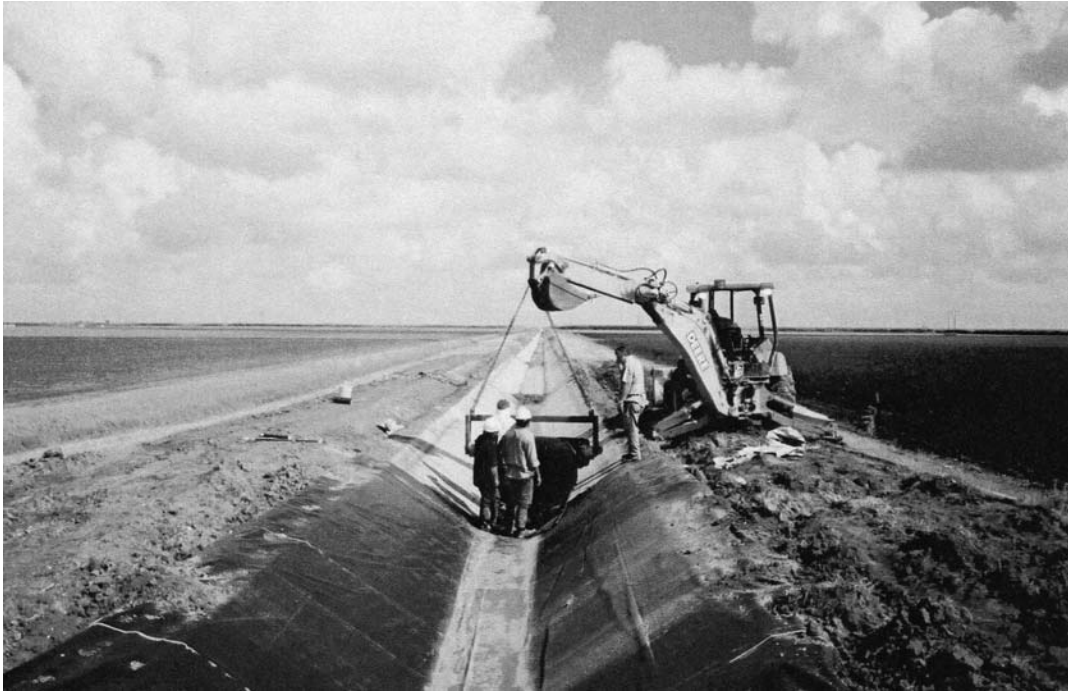
Photo 1. Typical Condition of Deteriorated Concrete Canal Section
