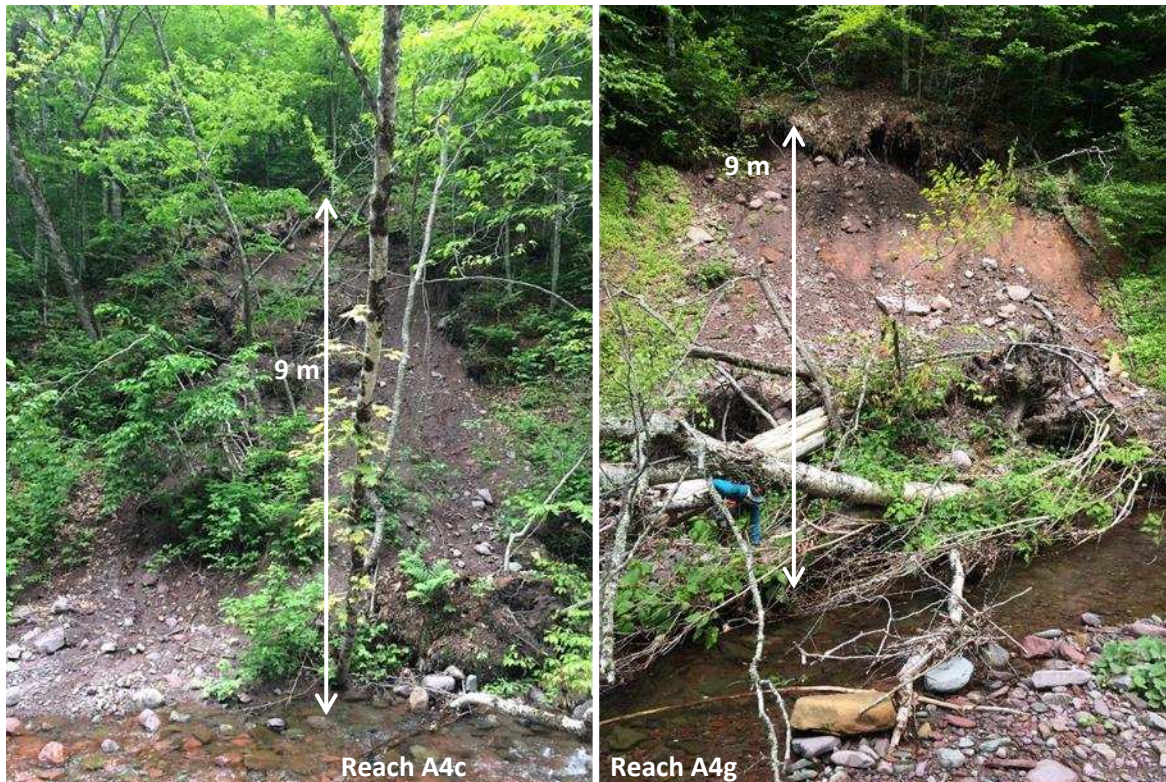
Figure 5. Examples of major hillslope failures in Biscuit Brook
