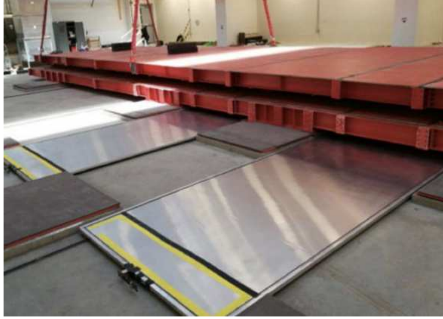
Figure 4.3: Bottom CRT installation below the ICARUS cryostat.
