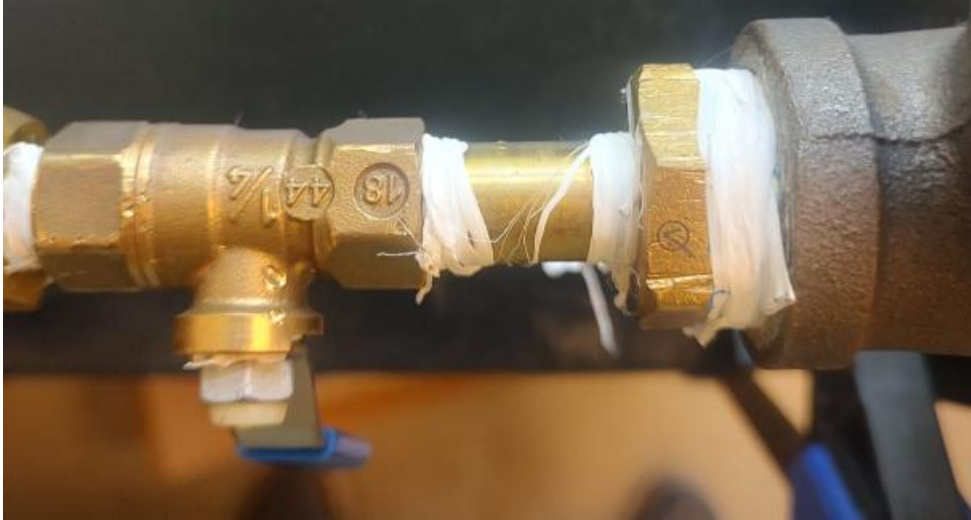
Figure 54- Connection too TEE from ball valve
