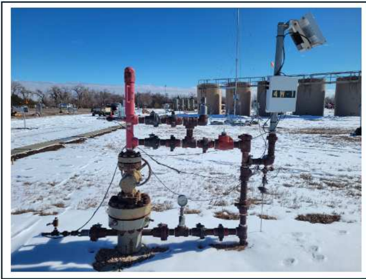
Figure 1.2: Example of oil and gas wellhead.
