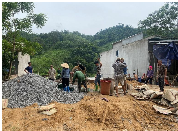
Figure 3.5: A group of villagers in Tat laying the foundation of a new concrete home (Thomas Chittenden)
