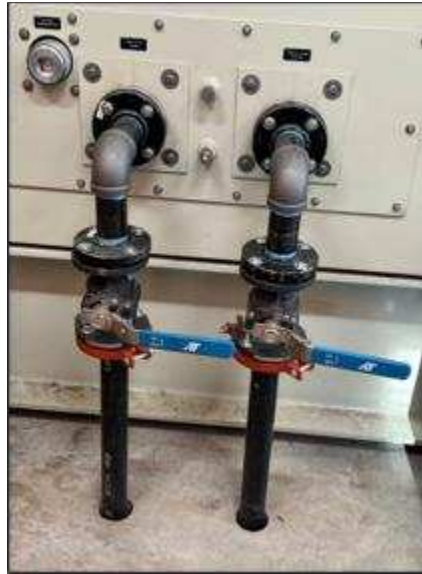
Figure 5.3 Piping to lube oil system heat exchanger.
