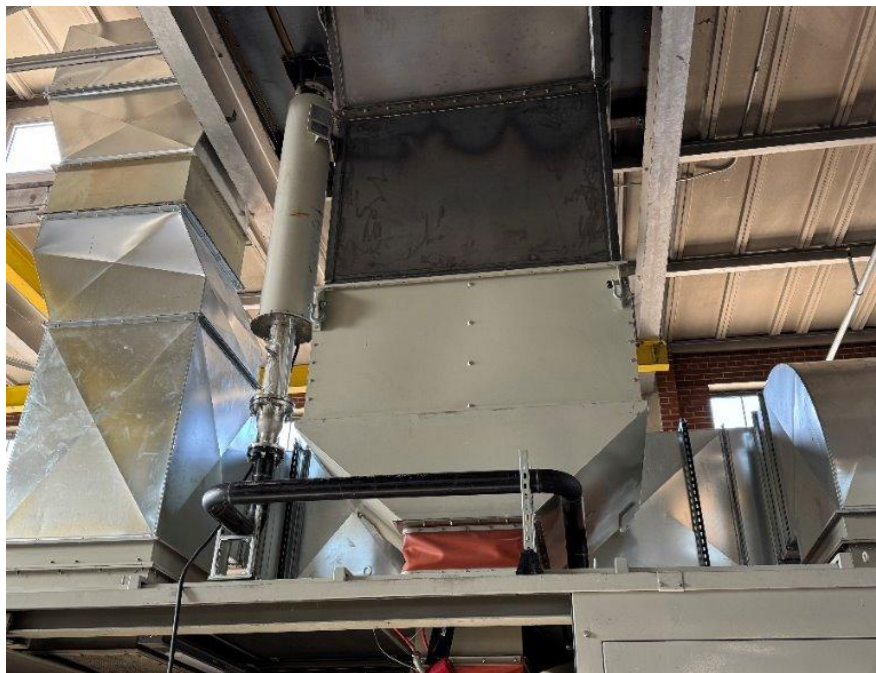
Figure 5.6 Lube oil demister installation with the flame arrester outside the building.
