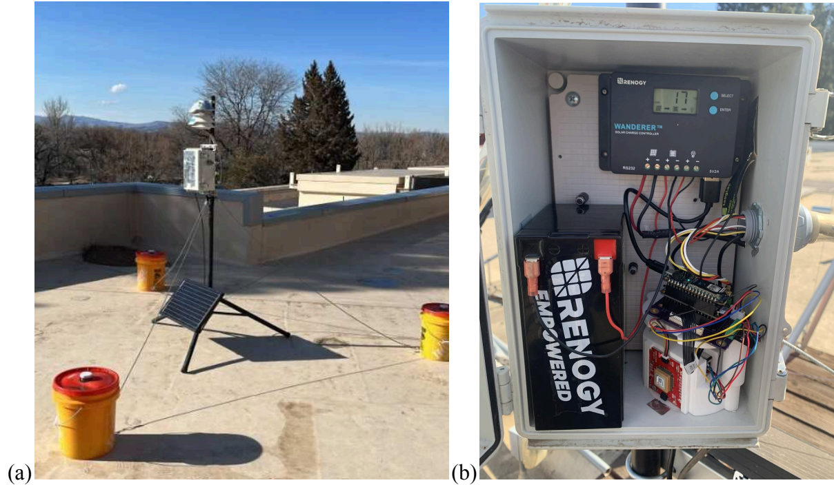
Figure 2.1.1 a) Full standing image of the VOZbox on the rooftop of Powerhouse, CSU. b) Image of the internal components of the control box, which houses the battery, charge controller, PM sensors, GPS unit, Boron, and PCB.
