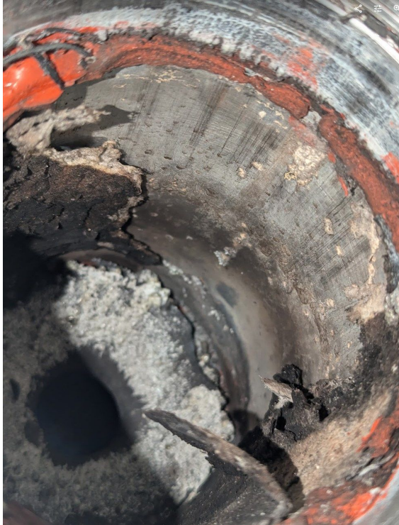
Figure 4.26: Combustion chamber liner condition after test fire
