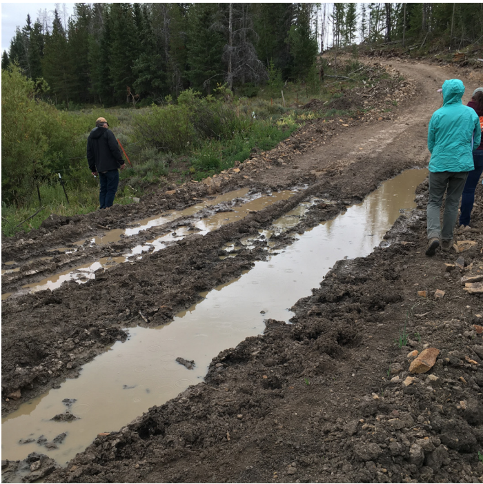
Figure 6: Team members observe inadequate drainage at a stream crossing. Photo: Diana Selby, CSFS
