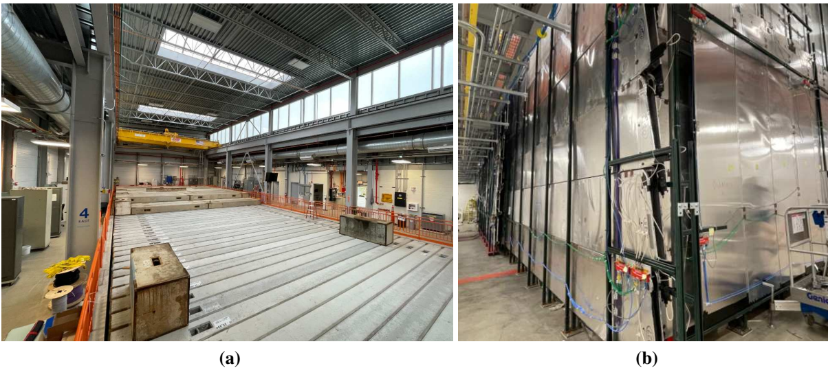
Figure 5.6: Left: The ICARUS concrete overburden during installation. Right: The ICARUS side CRT. Photos from the ICARUS collaboration.
