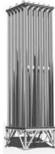
Figure 37: Nitrogen ambient air vaporizer. [33]
