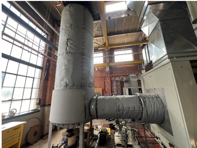
Figure 66: Image of exhaust system insulated with insultech blankets.
