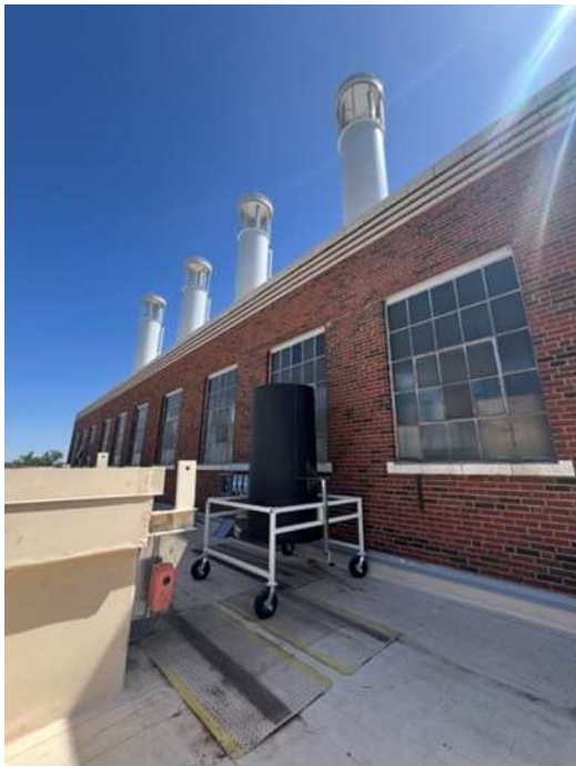
Figure 64: Mobile cart for raising and lowering exhaust stack.
