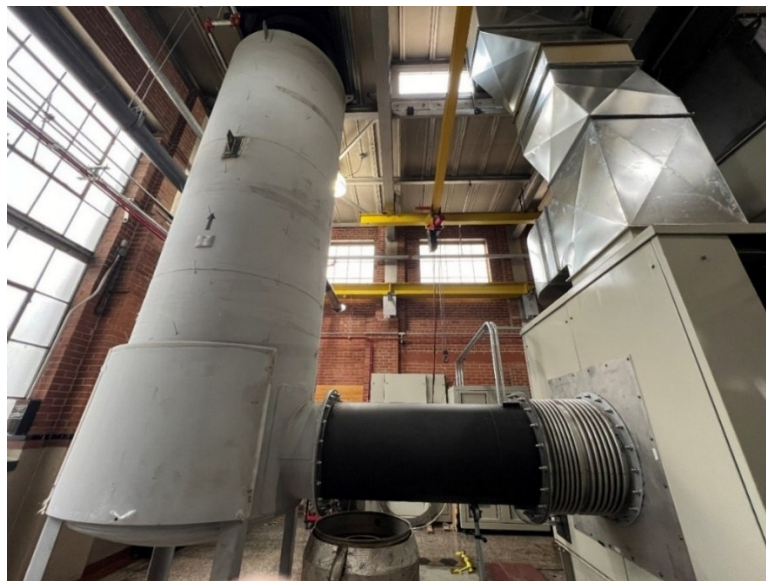
Figure 41: Internal building exhaust system comprised of expansion bellows, exhaust pipe extension, and silencer.
