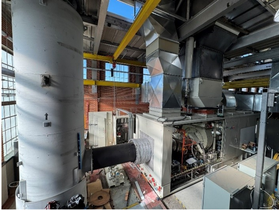
Figure 12: Solar Centaur 40 3.5 MWe gas turbine engine in research facility located at CSU powerhouse energy campus.
