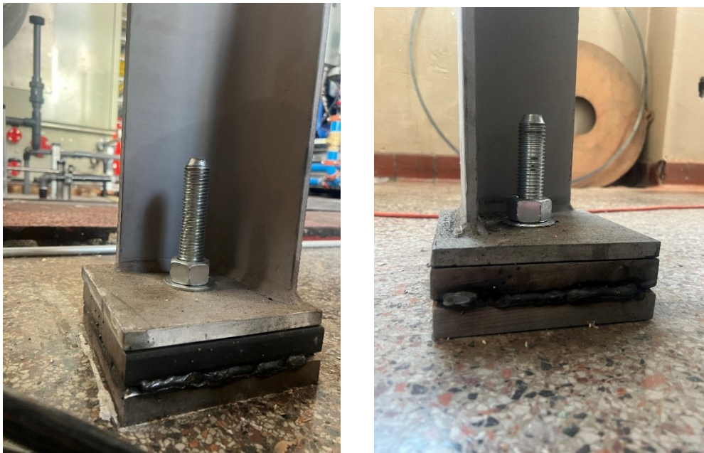
Figure 49: Two-inch shims under silencer feet, required to lift the silencer to match concentricity of the turbine exhaust, as the GT package was installed on 2 inch slabs, raising it above concentricity.
