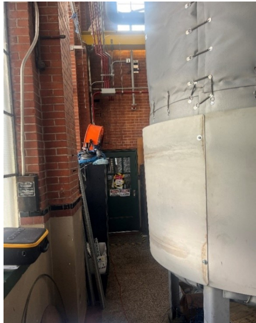
Figure 42: Silencer final position from south wall of research facility, maintaining standard 36 inches required for passageways.
