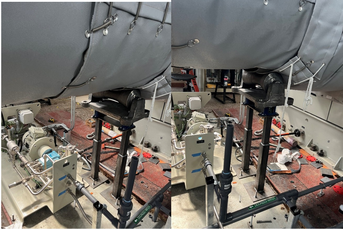
Figure 58: Images of installed Exhaust pipe extension support.
