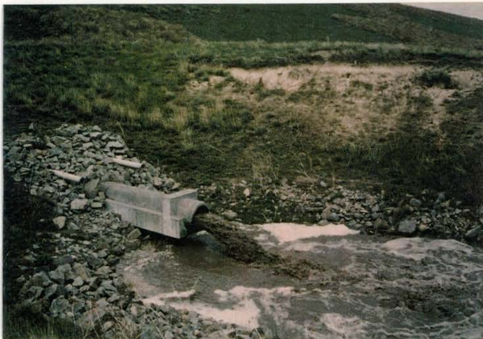
Figure 6.9 - Outlet works of Dam SS-3 after storm on June 11, 1998.
