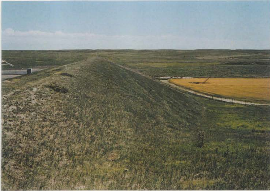
Figure 6.6 - View looking east across downstream face of dam SS-3 showing winter wheat crop at base of dam.
