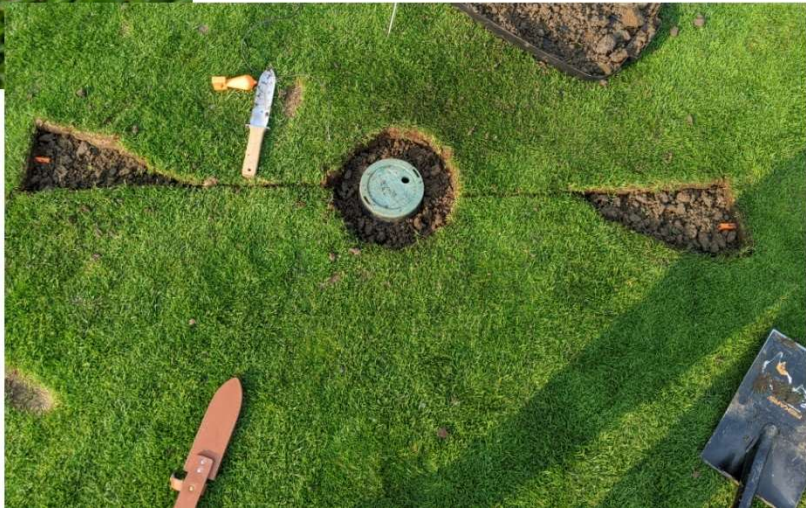
Figure 15. Demonstration of IoT Measurement Station before being covered up in the Fairway and side-view showing valve-box placement.
