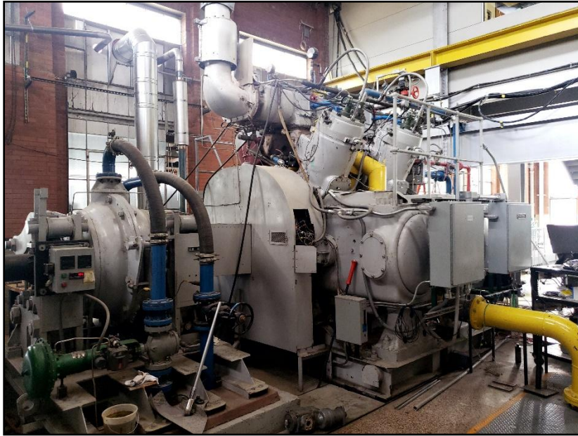
Figure 3-2 GMV-4TF engine housed at the Powerhouse Energy Campus, Colorado State University
