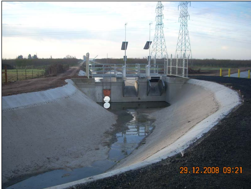
Figure 4. OID Diversion Structure - Post Rubicon Gate Installation
