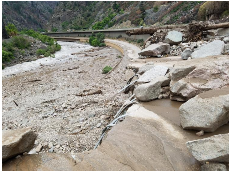
Photo of I-70 in Glenwood Canyon from Colorado Department of Transportation: https://twitter.com/ColoradoDOT/status/1421978755170410501
