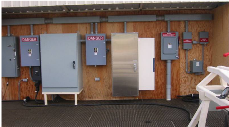
Figure 5. Electrical supply for the motor testing
