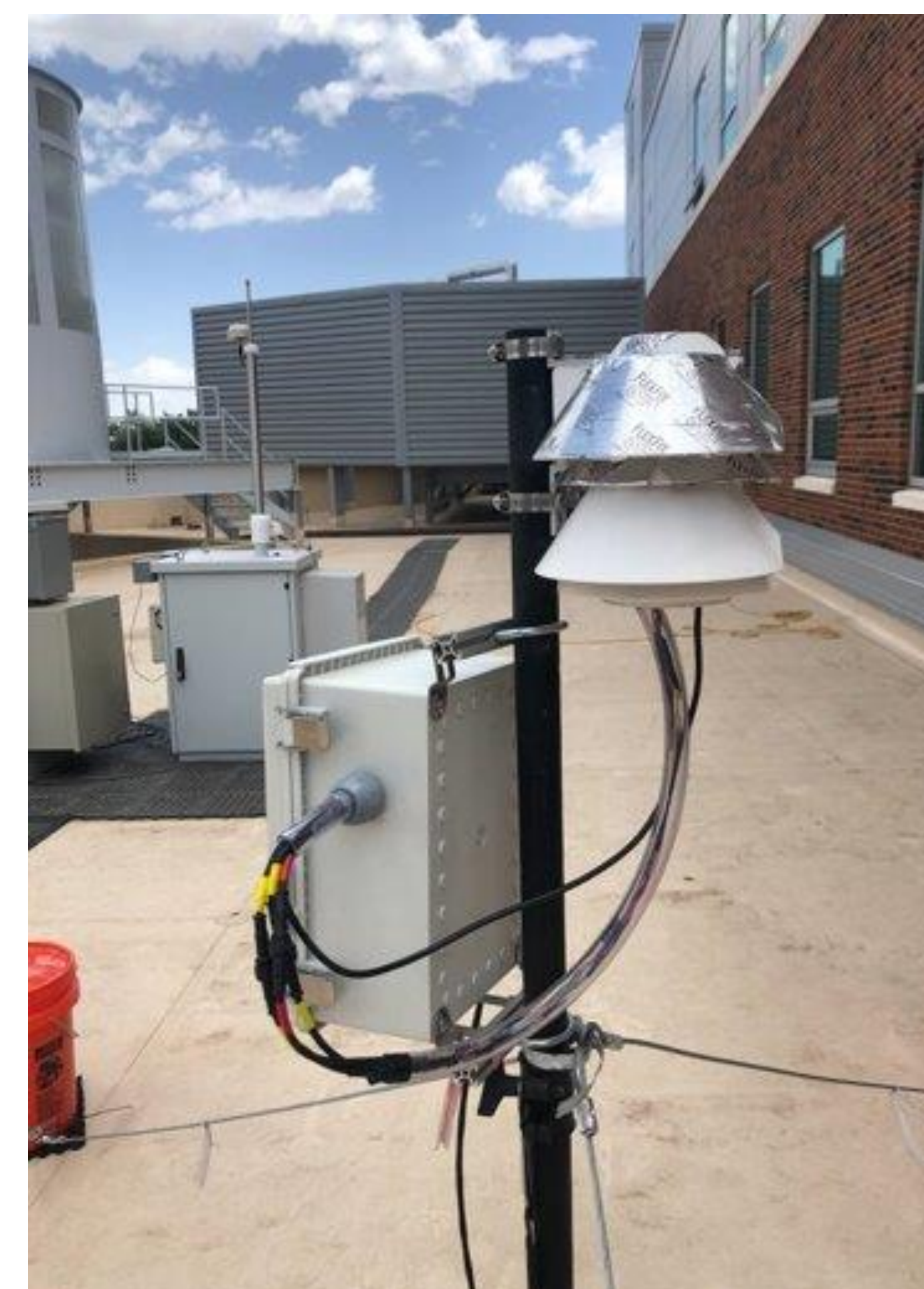
Figure 2: MOOS2A_1 on the Powerhouse rooftop. Pictured are the guy wiring and weatherproofing modifications.
