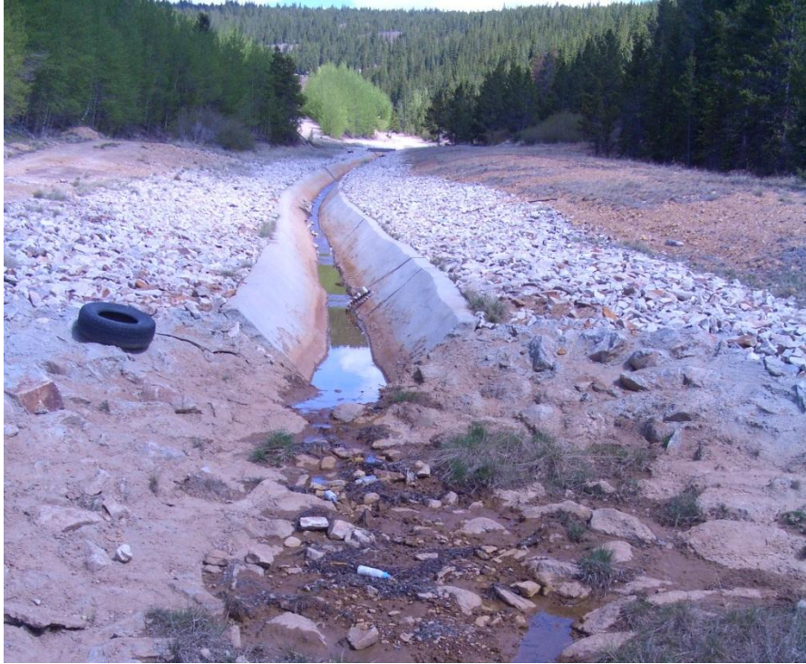
Figure C-5: View upstream from CG-1. California Gulch is a concrete-lined trapezoidal channel floor approximately 1.5 miles above the CG-1 gauge.
