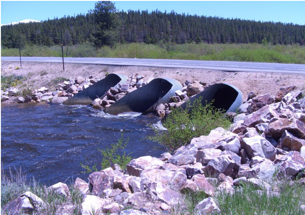
Figure C-60: Arkansas River at County Road 4. View of culvert inlets from right looking southwest.
