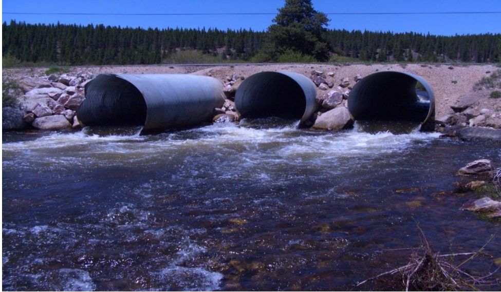
Figure C-63: Arkansas River at County Road 4. View of culvert outlets from left bank looking northwest.
