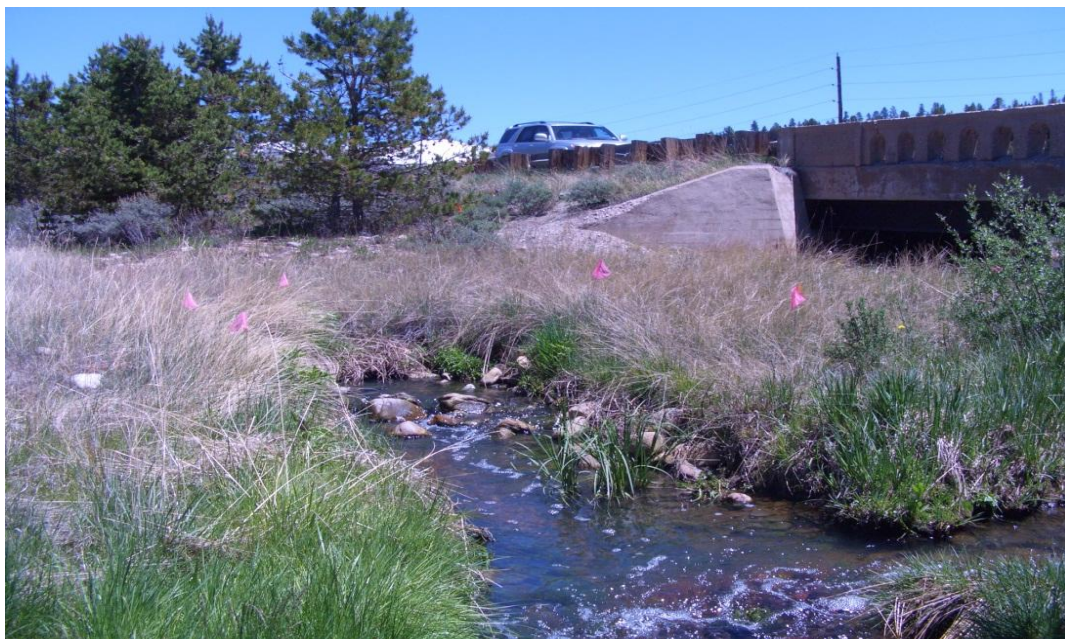
Figure C-46: WWTP discharge culvert downstream of US-24 bridge. Pink flags are CDOT wetland delineation.
