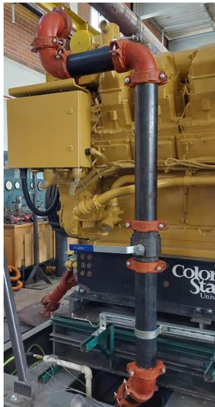
Figure 64. Jacket water-out line highlighting the ball valve for manual shut-off.
