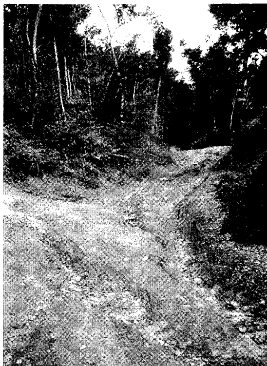
Figure 2. Example of a steep road segment near Bordeaux Mountain with a deeply-rilled travelway.
