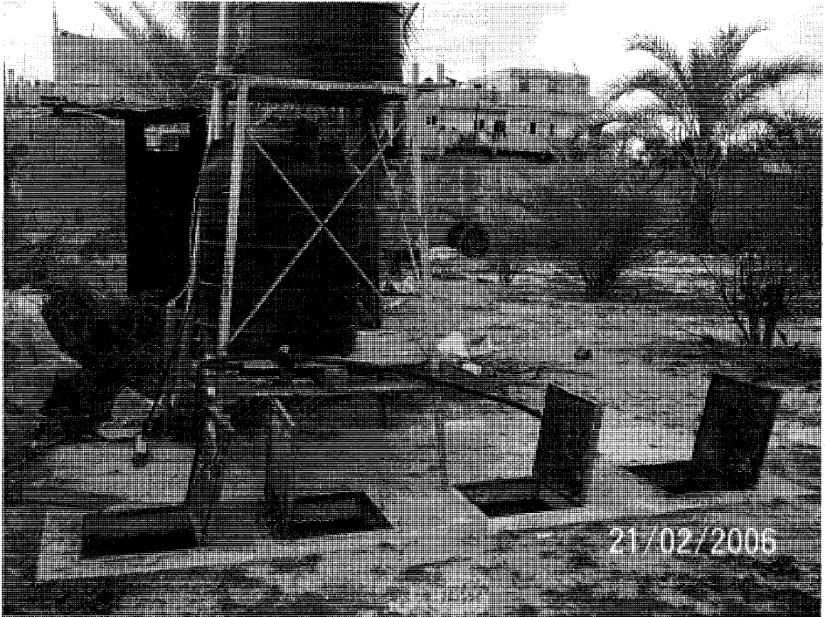
Figure 5.2 A constructed graywater system used by the Agricultural Development Society in Palestine along with the openings of each treatment chamber
