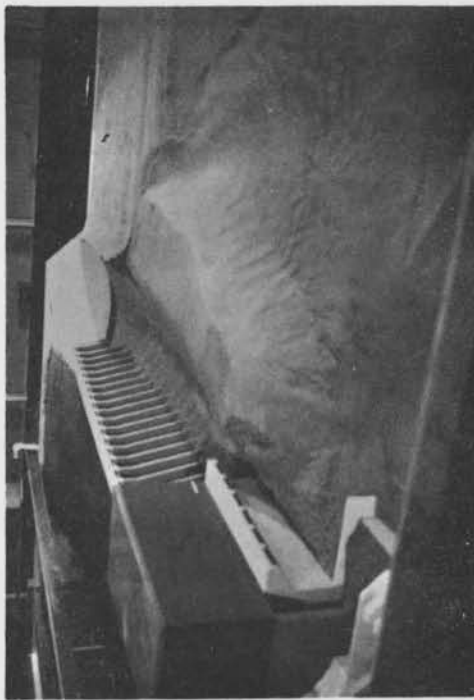
D Scour Conditions Downstream from North Abutment
