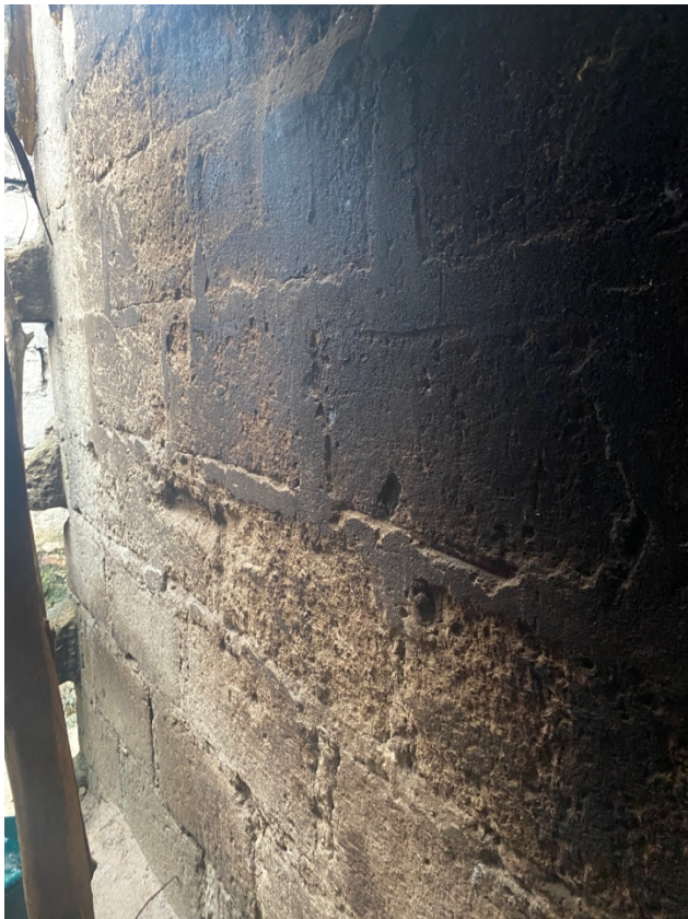
Figure 6: Image of the smoke damage from a TSF on a kitchen wall (DeGrandpre, 2025).
