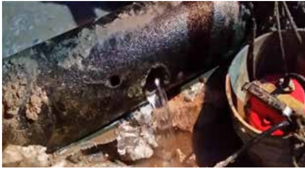
Aging infrastructure before replacement. Photo courtesy of the Town of Silt and DOLA.
