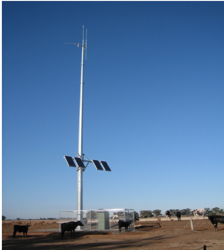
Figure 5. Communications Node Site
