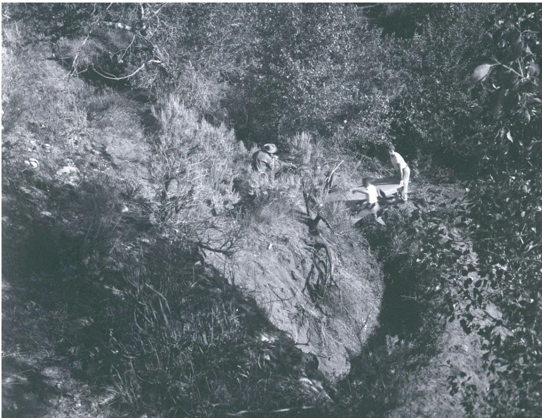
Figure 15 – Construction of the trackway at the beginning of 1948 season. Looking west. (ARC.DNM04_001_1833)
