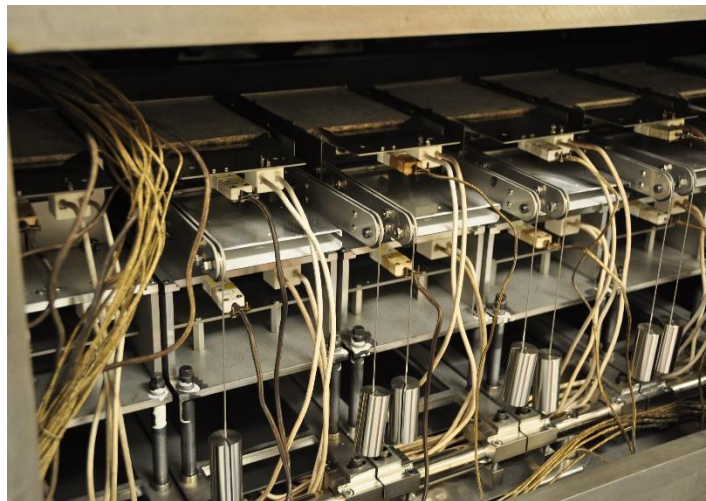
Figure 19 Top: Picture of the ARDS; Bottom: Picture of the CSS sources inside the ARDS.
