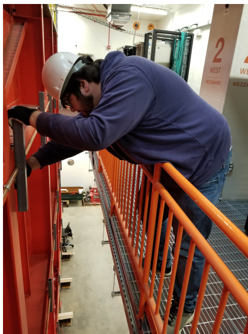
Figure 2.38: Installation of the fiberglass pieces that would hold the Unistrut support posts to the warm vessel.
