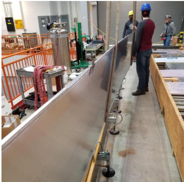
Figure 2.40: During the West Center/Rolling Wall installation, modules were initially loaded one at a time at the loading dock.
