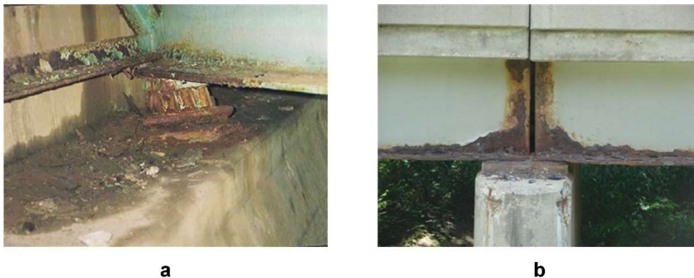
Figure 2.5 – Corrosion of a) rocker bearing (Wells et al., 2017) and b) steel girders end (CTT, 2017)
