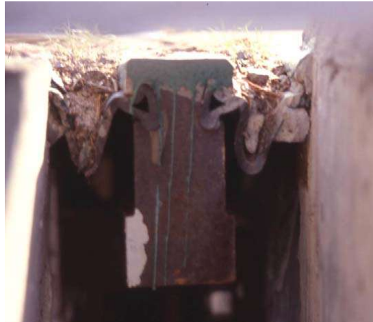
Figure 2.2 – Debris in expansion joint (Chen, 2008)
