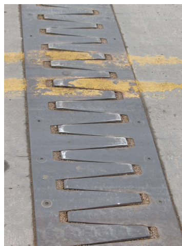
Figure 2.3 – Finger joint clogged by debris on bridge B-16-FM (Rager, 2016)
