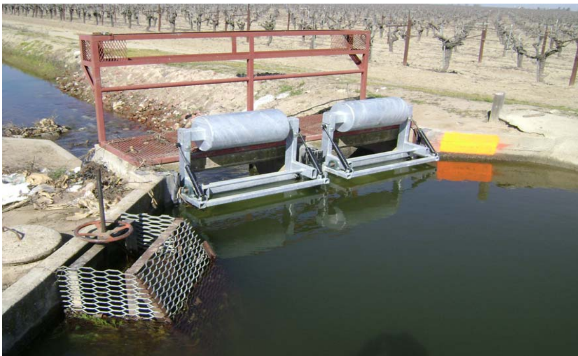
Figure 2. Typical Weir Retrofitted with ITRC Flap Gate
