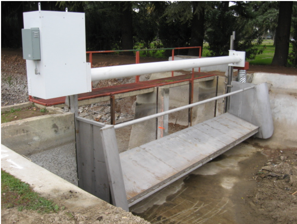
Figure 5. Langemann Gate Used to Automate Headgate
