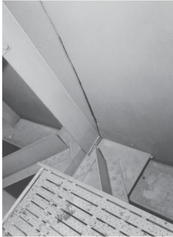
Fig. 2.12. The Lafayette St. Bridge fully fractured girder (Connor et al. 2005)
