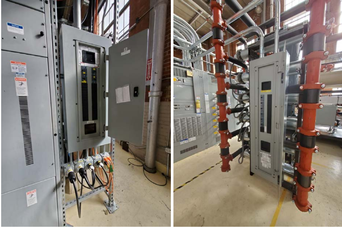
Figure B-7 Test facility electrical supplies
