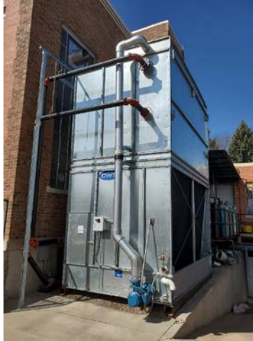
Figure 4-5 Condenser loop cooling tower
