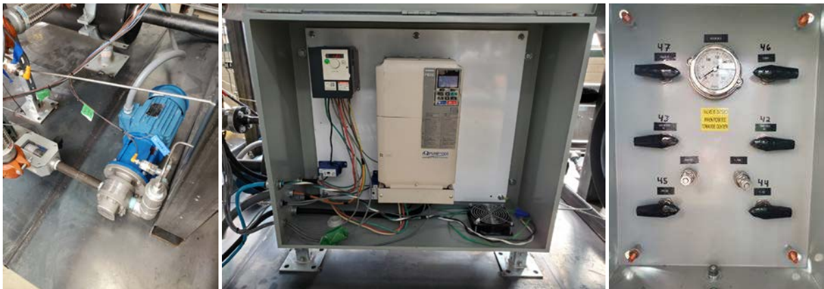
Figure B-2 (Left to Right) Fluid management pump, variable frequency drives, and fill/drain station
