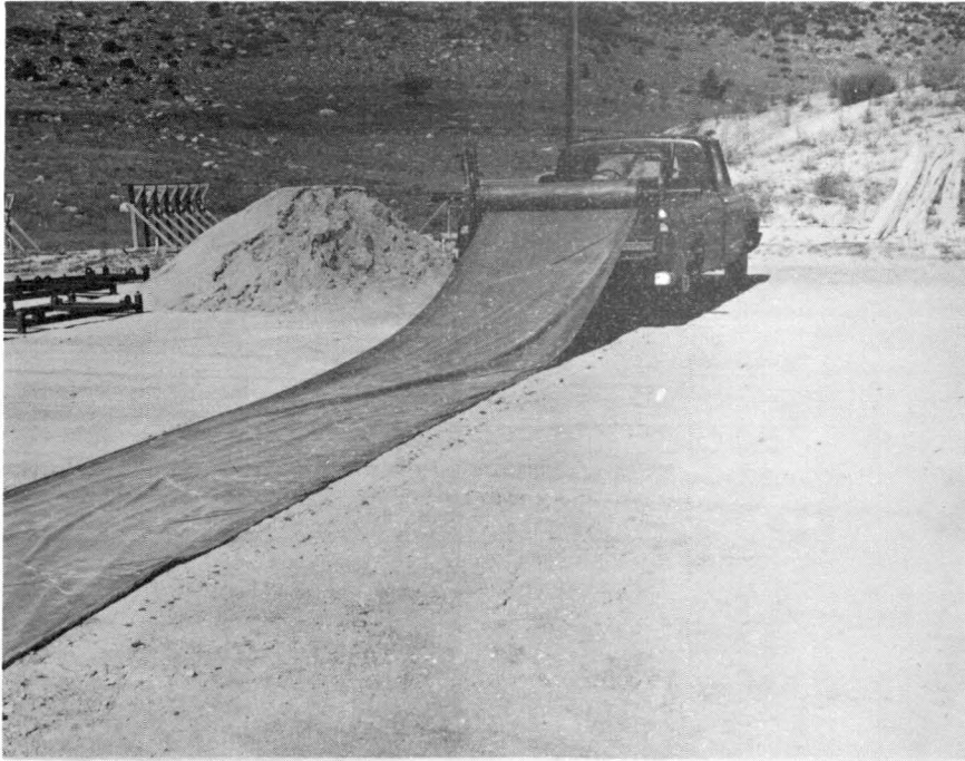
Fig. 7 - The 1000-pound roll of butyl rubber was unrolled from a pick up truck.
