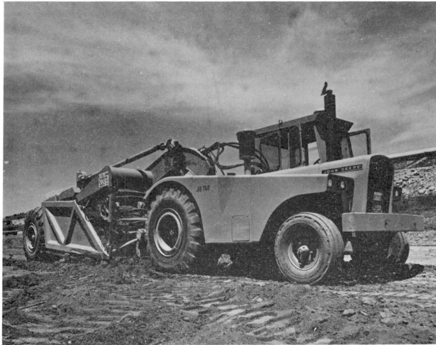
Fig. 1 - A layer of selected fill material was hauled into the watershed area. This provided a subbase for the final grading.
