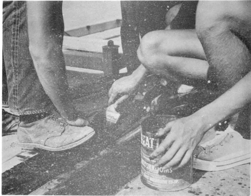
Fig. 9 - The 6-inch wide overlapping edges of the rubber were thoroughly cleaned and treated with joint cement.
