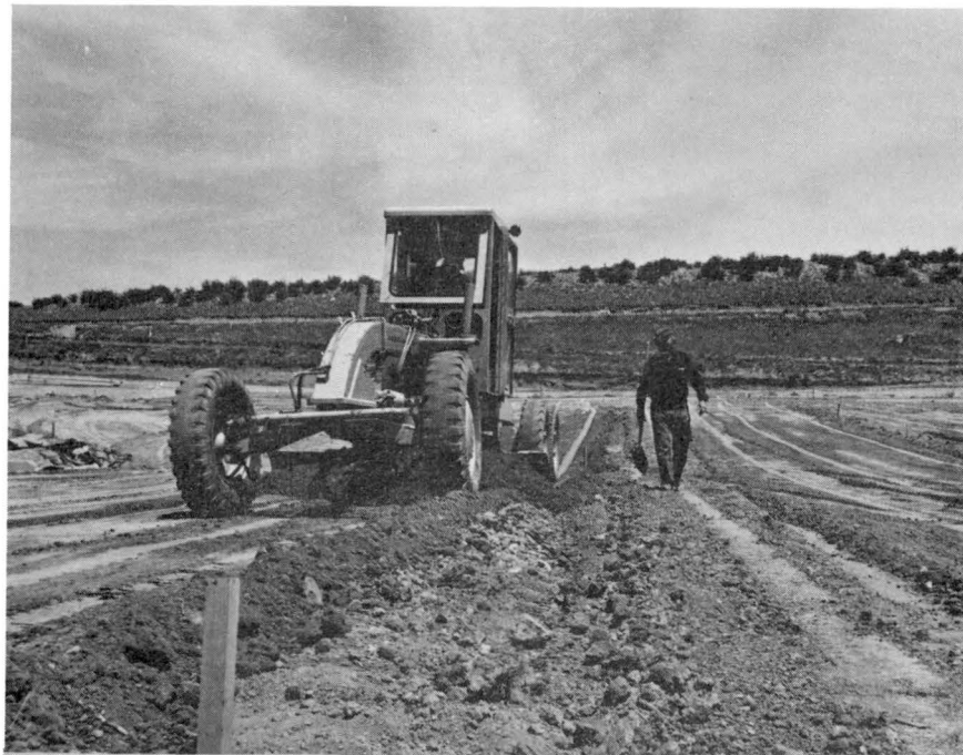
Fig. 2 - The watershed surface was graded to a smooth surface approximately 1/2 inch below final desired grade.
