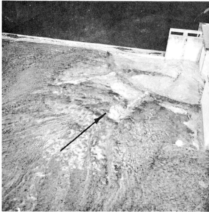
Fig. 10. Modification B. Q = 25 c.m.s. Sediment is shown entering settling basin with sluice gates closed.
