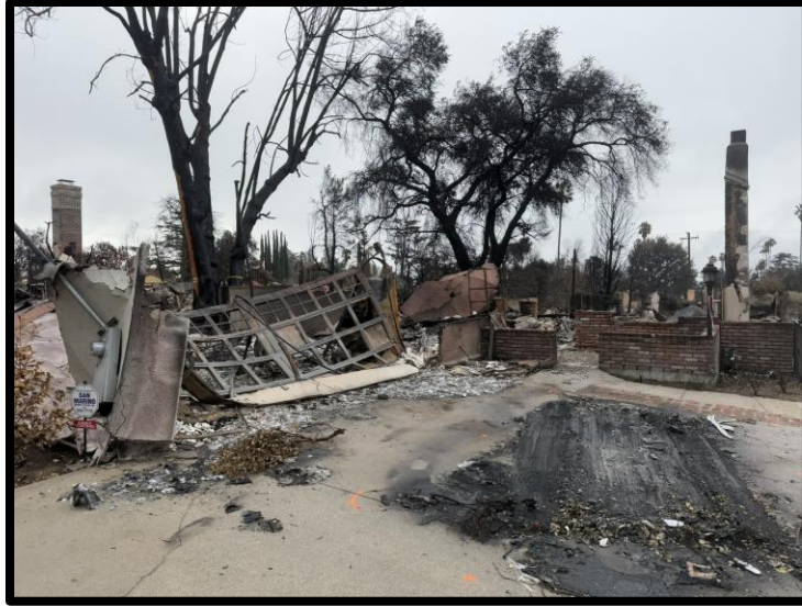
Figure J6. Photo of one of the destroyed properties that we sampled from.
