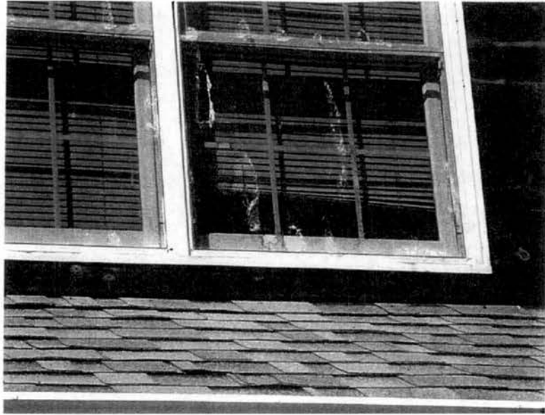
Figure 4.2: Torn window screens in Parker.
