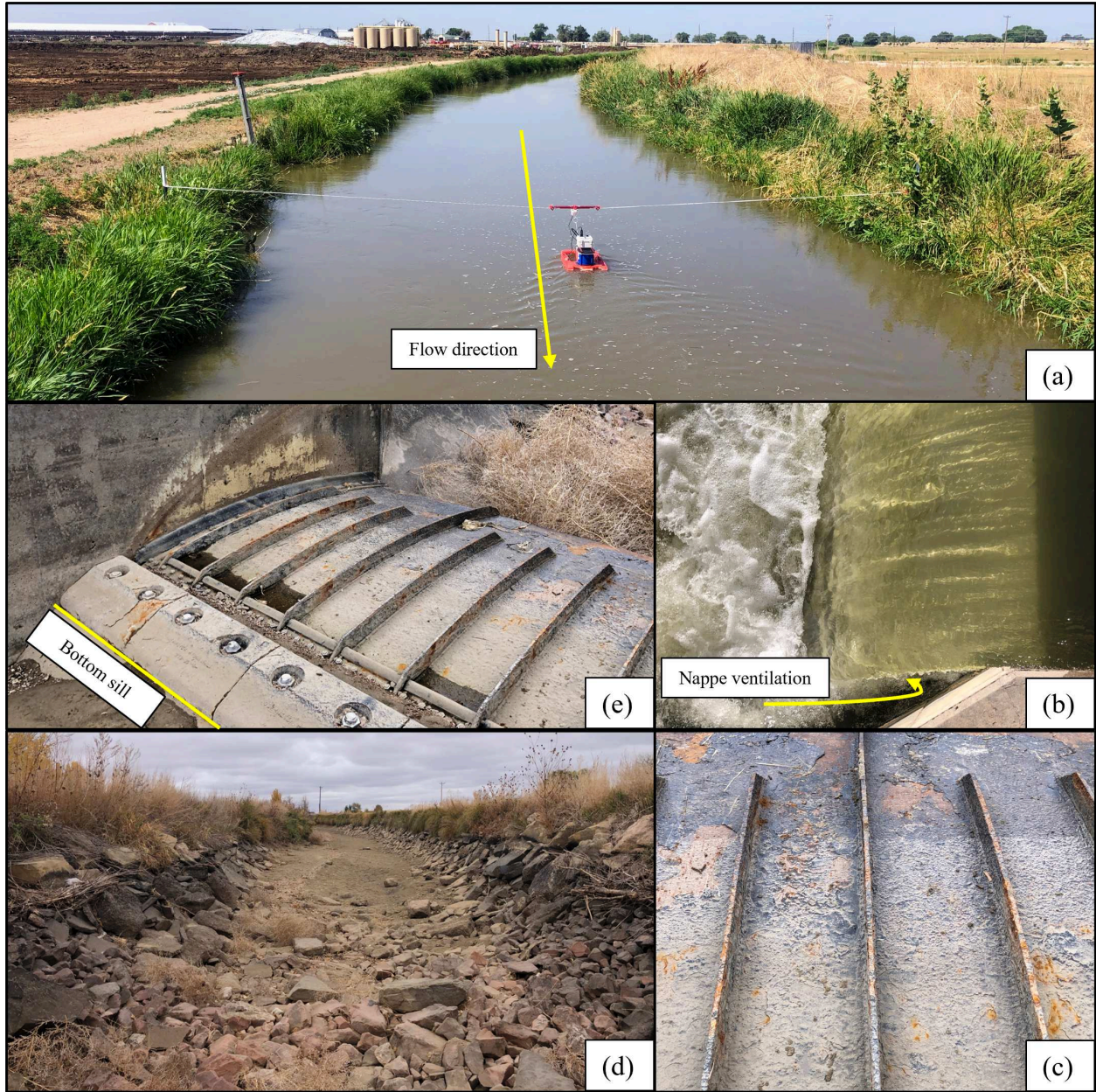
Figure B.3: Site characteristics at Weir C. a) Approach flow conditions looking upstream, some curvature in channel approach can be seen. b) Evidence of aeration due to divergent sidewalls downstream of crest. c) Corrosion on surface of weir blade. d) Rip-rap placement downstream of weir to dissipate energy. e) Mounted weir structure on bottom concrete sill.
