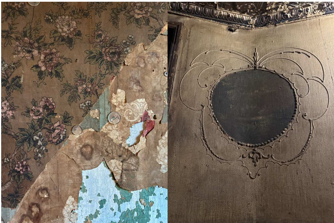
Figure 6 Peeling wallpaper & Figure 7 Soot covered wall art. Photograph by Author
