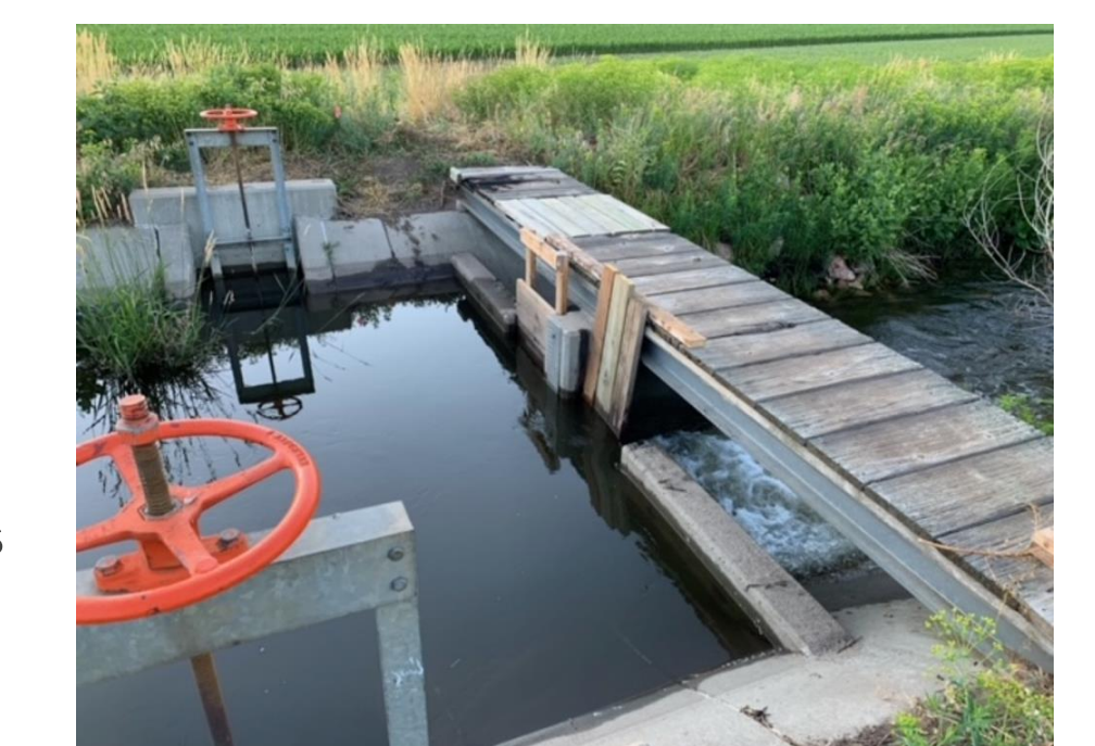
The headgate was used to control flow of water to the irrigation ditches
