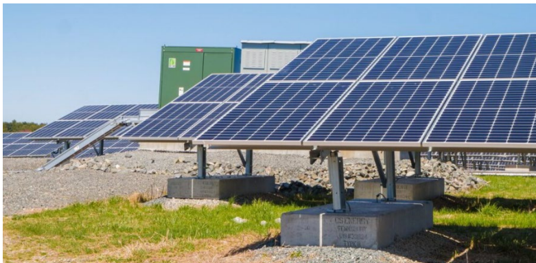
Ballast-Mounted Solar Array atop the Rocco Landfill, Tewksbury, MA.
