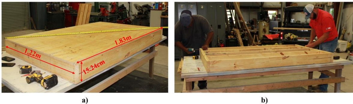
Figure 6-1: a) construction of wood barriers and b) constructed wood barrier with no sand.
