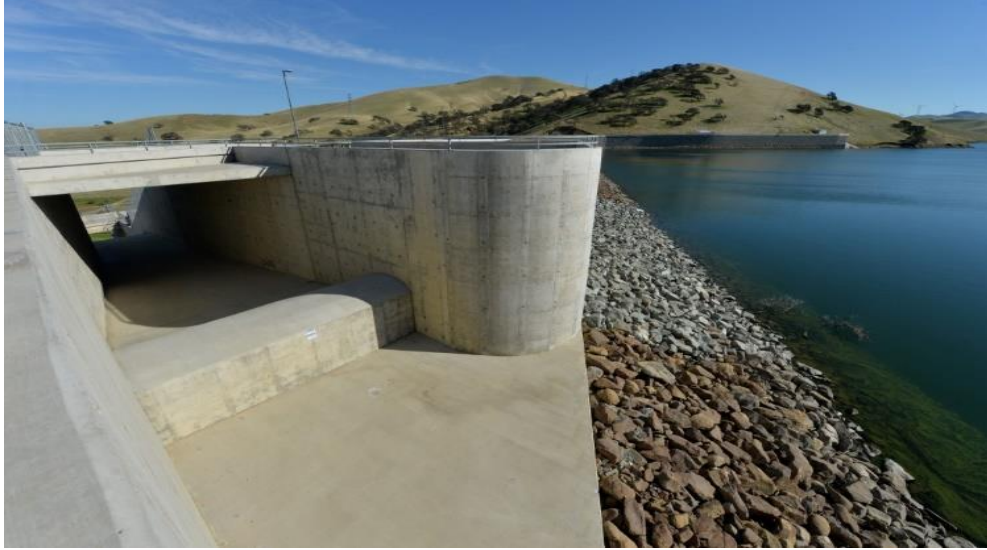
Figure 1-1. The present ogee-shaped weir set back from the circular abutments of the existing Los Vaqueros Dam (view shows unheightened dam).
