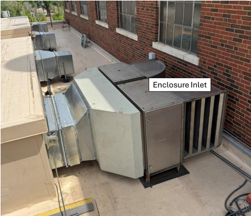
Figure 23: Enclosure Ventilation Inlet Duct.
