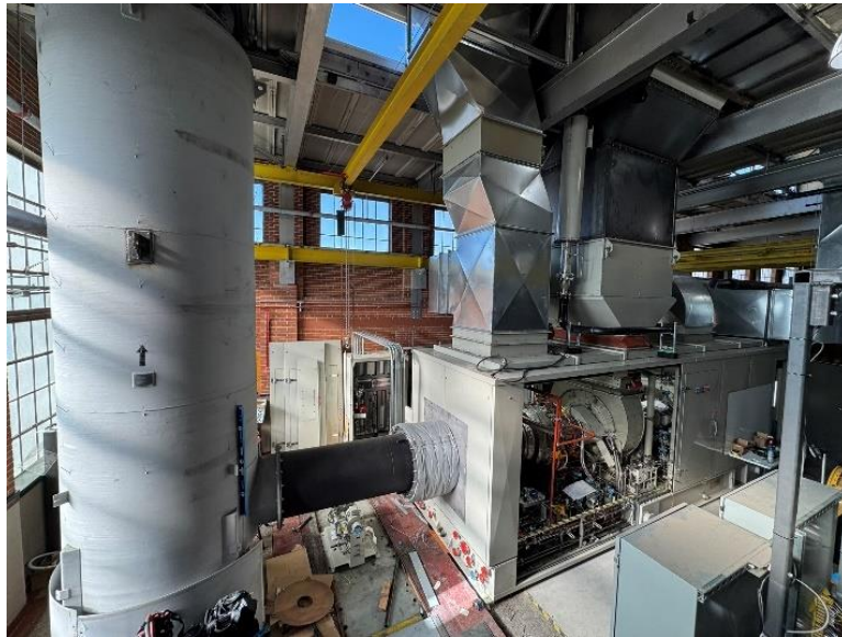
Figure 8: Solar Turbines Centaur 40 Gas Turbine Located in CSU Powerhouse Research Campus.
