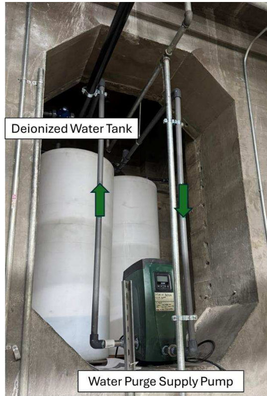
Figure 25: Water Purge Supply Pump.
