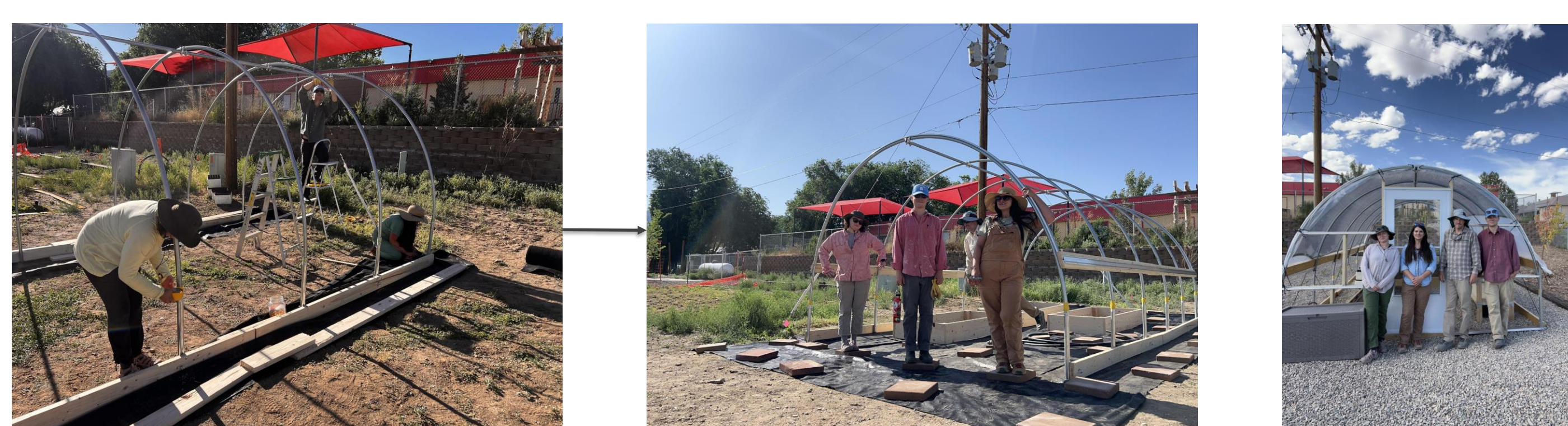
Early, middle, and late stages of work throughout two trips to the Ute Mountain Ute Reservation on a high tunnel for Kwiyyagat Community Academy
